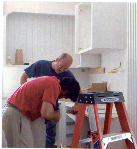
Kitchen cabinets are installed by Alex Stivala, owner of Carpen House, and a staff installer.
